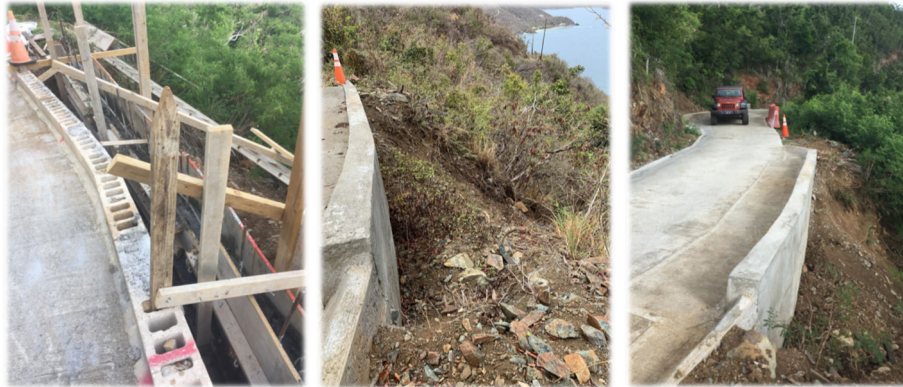
Figure 2-32. Freeman's Ground, St. Johns, USVI retaining wall for road stabilization. Source: Coral Bay Community Council
