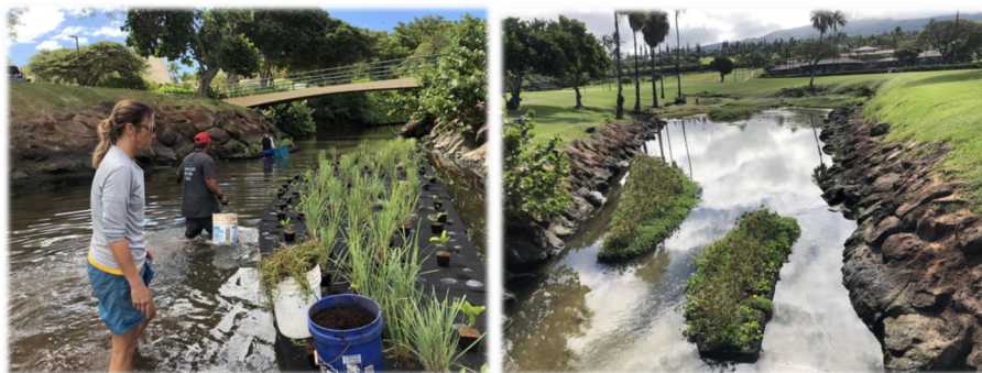
Figure 2-38. Example of an under construction (left) and finished floating wetland (right). Source: West Maui Ridge to Reef
