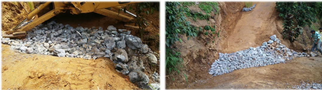
Figure 2-36. An example of swale construction in Puerto Rico. Source: Protectores de Cuencas
