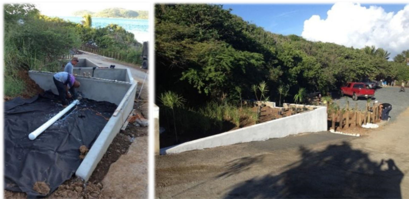
Figure 2-39. Building constructed wetland (left) and finished wetland (right). Source: Protectores de Cuencas
