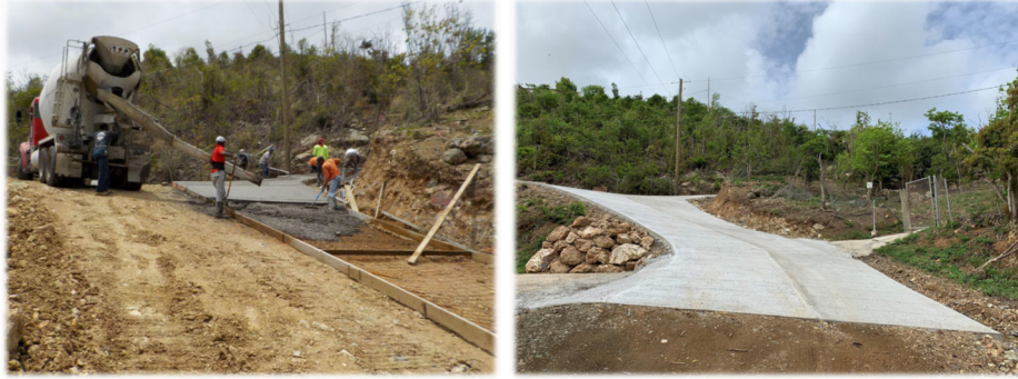
Figure 2-31. Gerda Marsh road stabilization on St. Johns, USVI. Source: Coral Bay Community Council
