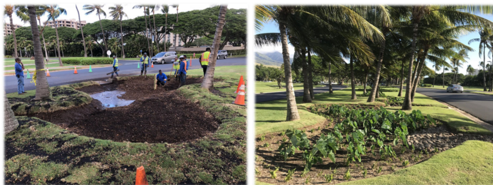
Figure 2-34. Constructing (left) and finished (right) bioretention area in West Maui. Source: West Maui Ridge to Reefs
