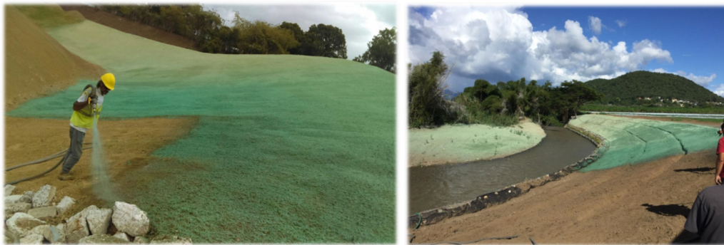
Figure 2-30. Hillside hydroseeding in Puerto Rico. Source: Protectores de Cuencas
