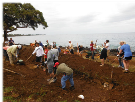
Figure 2-35. Constructing a rain garden in West Maui. Source: West Maui Ridge to Reefs
