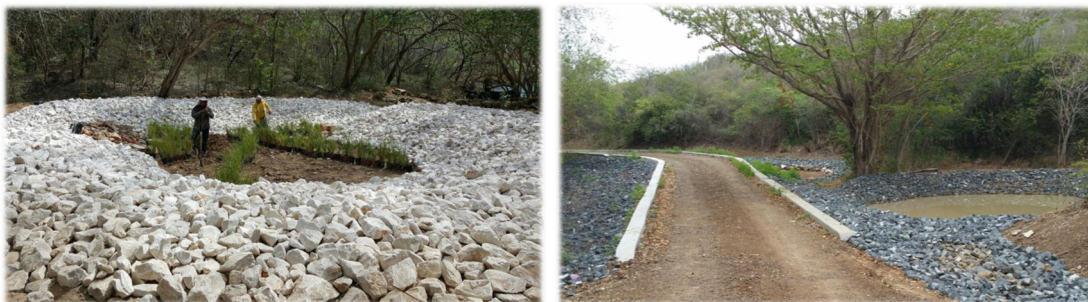
Figure 2-37. Examples of constructed stormwater ponds in Puerto Rico. Source: Protectores de Cuencas
